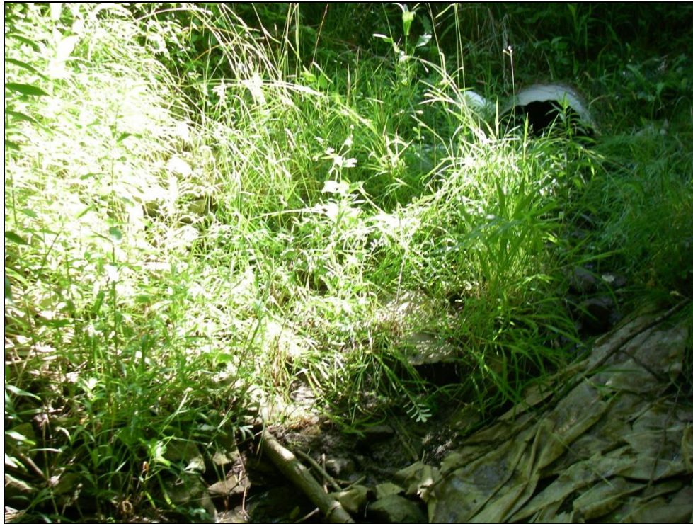
Photo 5: Youngstown Drain, looking northeast (upstream) towards E.C. Row to Huron Church Road eastbound to southbound off ramp culvert.
