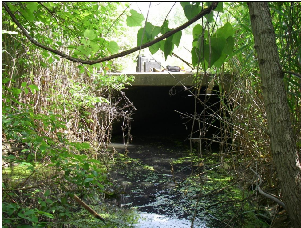
Photo 1: McKee Drain, looking southeast (upstream) towards the E.C. Row Expressway culvert crossing.
