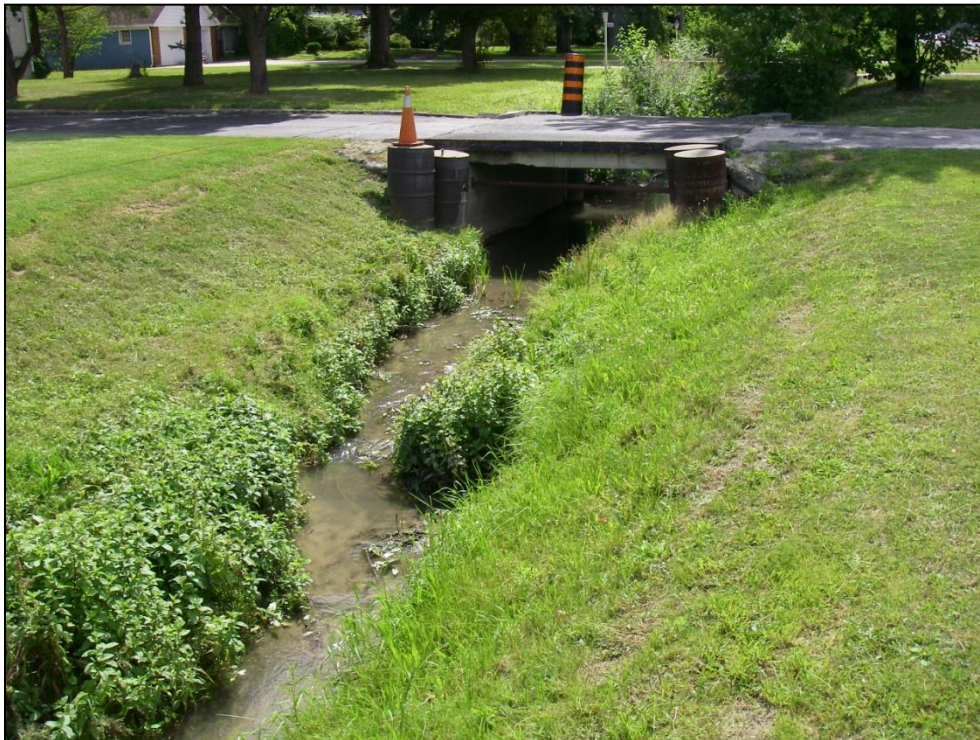
Photo 16: Wolfe Drain looking southeast (upstream) towards a driveway between Cousineau Road and Howard Avenue.
